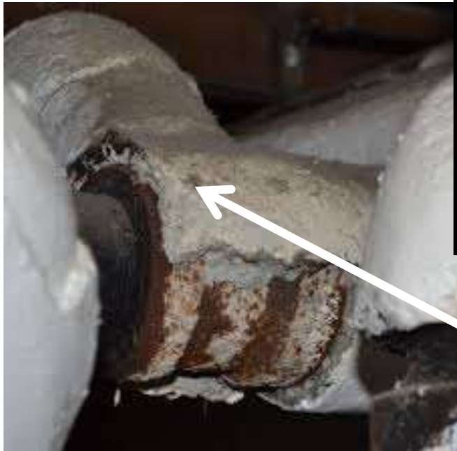
Asbestos insulation around a pipe
